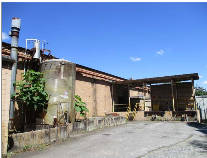
Photograph 35: View of east elevation of Catawba Complex including cistern and loading dock; looking northwest. (2017)
