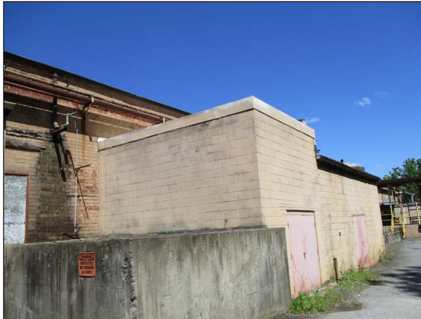
Photograph 34: View of concrete block addition on east elevation of Catawba Complex; looking northwest. (2017)
