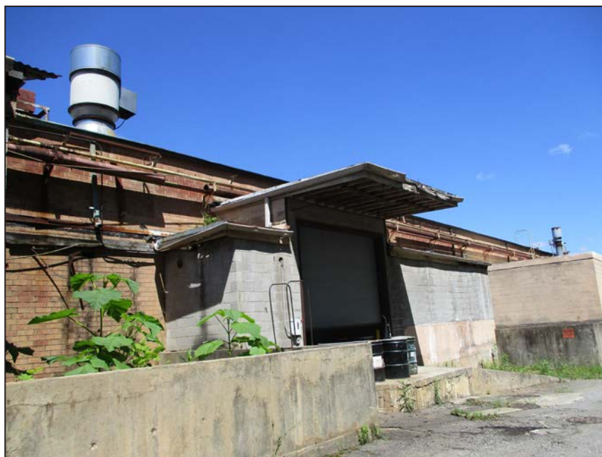
Photograph 33: View of loading dock on east elevation of Catawba Complex; looking northwest. (2017)
