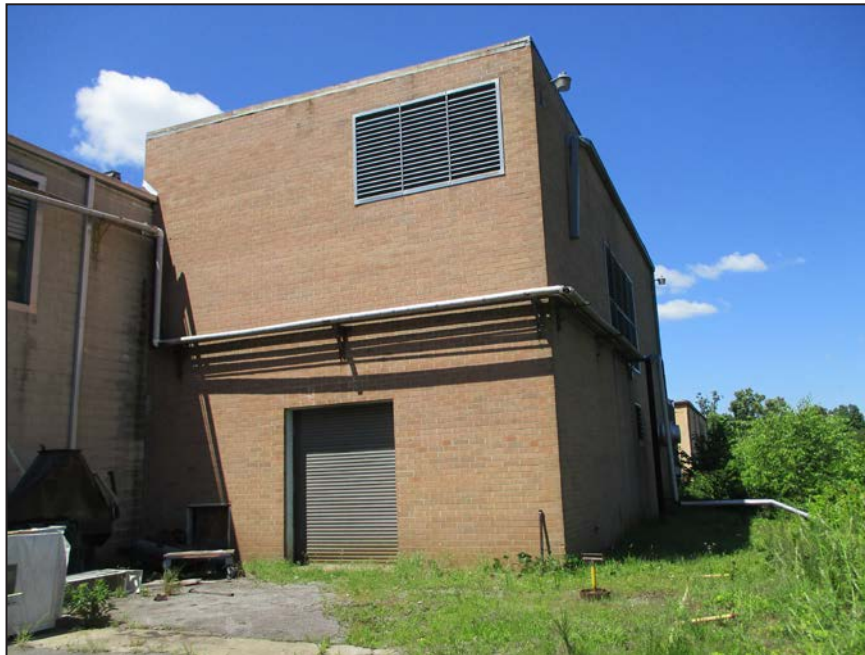
Photograph 28: View of addition off of north elevation of Catawba Complex; looking northwest. (2017)
